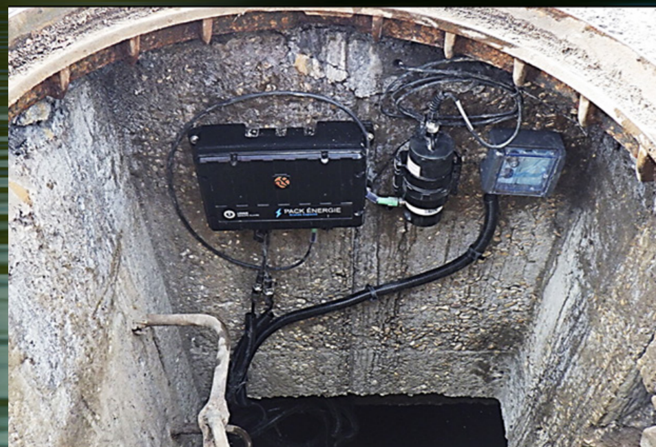
Figure 4: Data logger, battery pack, and programmer for the turbidity probe cleaning system of PC527-101 Sainte Hélène Thiers.
